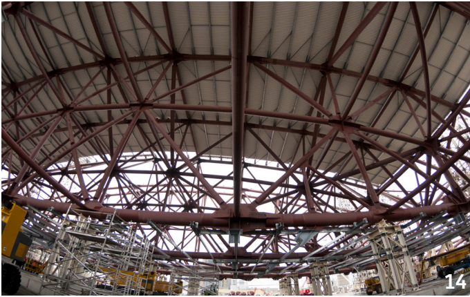
October 2012: The cladding starts with the installation of the purlins and complex wall system. - @Guillaume Daveau
